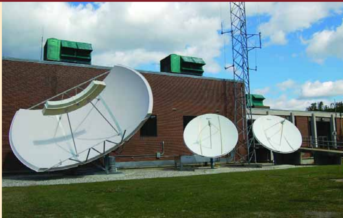
Satellite dishes behind Groton City hall are used to receive broadcast TV signals that are then made available to cable TV customers. Thames Valley Communications now serves more than 7,000 customers after being in full operation for just three years.
